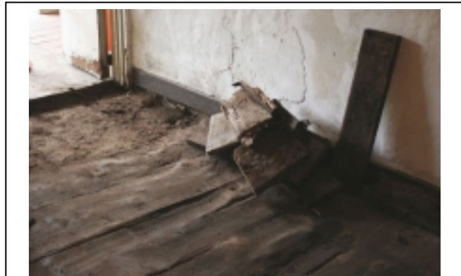
The rutted redwood plank floor at the threshold of the Museum entryway was so rotted by humidity that much of it had been reduced to the consistency of a wooden sponge. Photo © Ruben G. Mendoza, 2006.
