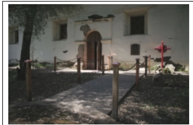
The crews from Trujillo Construction completed the replacement of the redwood posts and chain barriers in the Old Mission Cemetery in April 2006. Photo © Ruben G. Mendoza, 2006.
