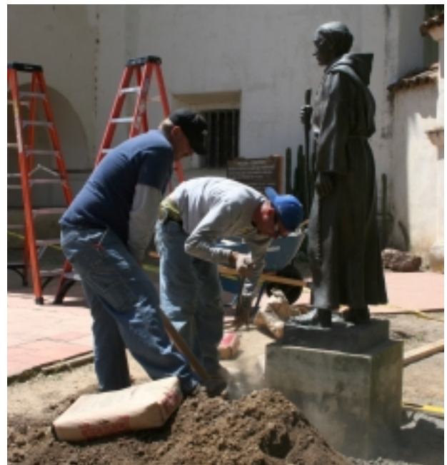
Killian Construction crew members reinstall the Serra statue at its new location adjacent the cemetery gateway on May 8, 2006. Photo © Ruben G. Mendoza, 2006.
