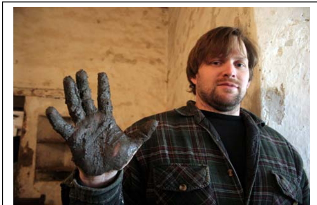
CSU Monterey Bay student and project crew member Gerald Jones recently worked to mud and lime coat interior walls in the Old Convento. Photo © Ruben G. Mendoza, 2007.
