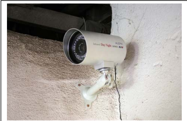
One of over 16 Aleph America Corporation Infrared Day Night cameras installed at Old Mission San Juan Bautista. Photo © Ruben G. Mendoza, 2007.
